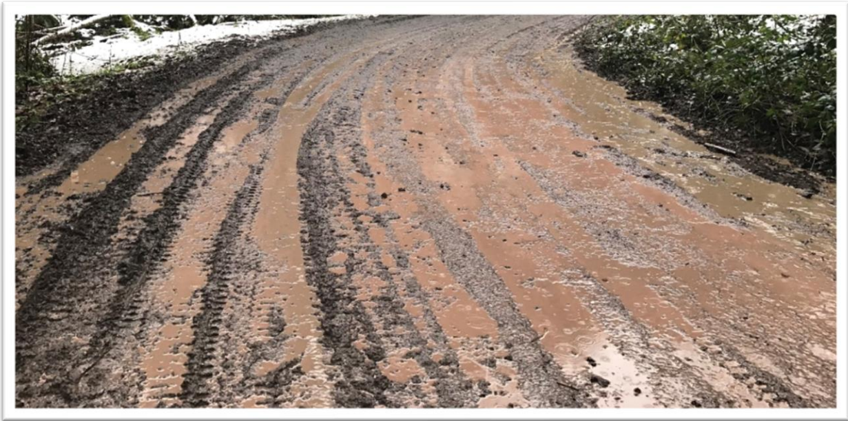
Photo 5. Road surface with a layer of mud.
