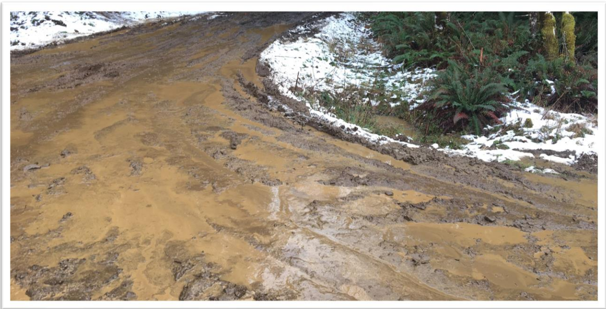
Photo 4. Road surface with a layer of mud.
