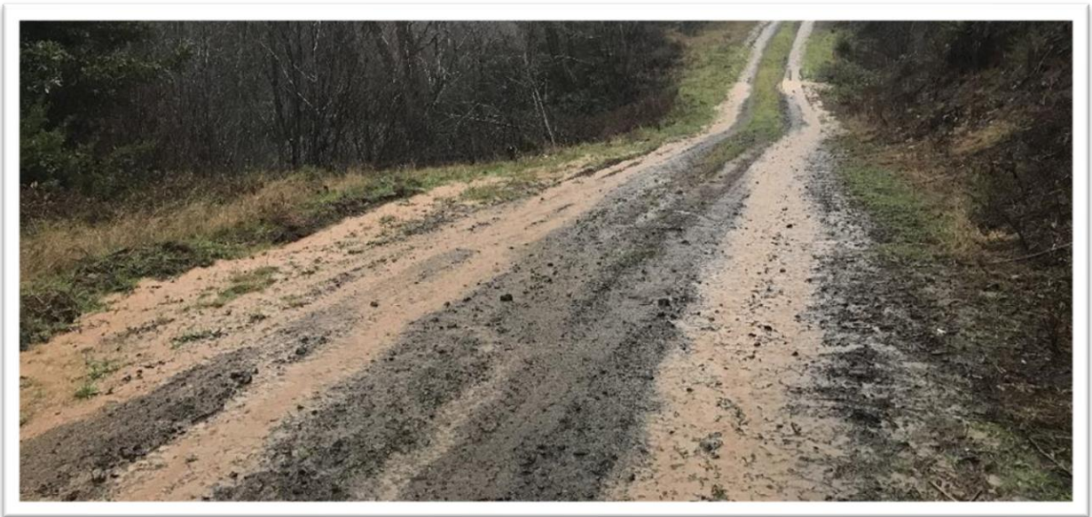
Photo 6. Rutted road, road shape does not move water off the road surface.
