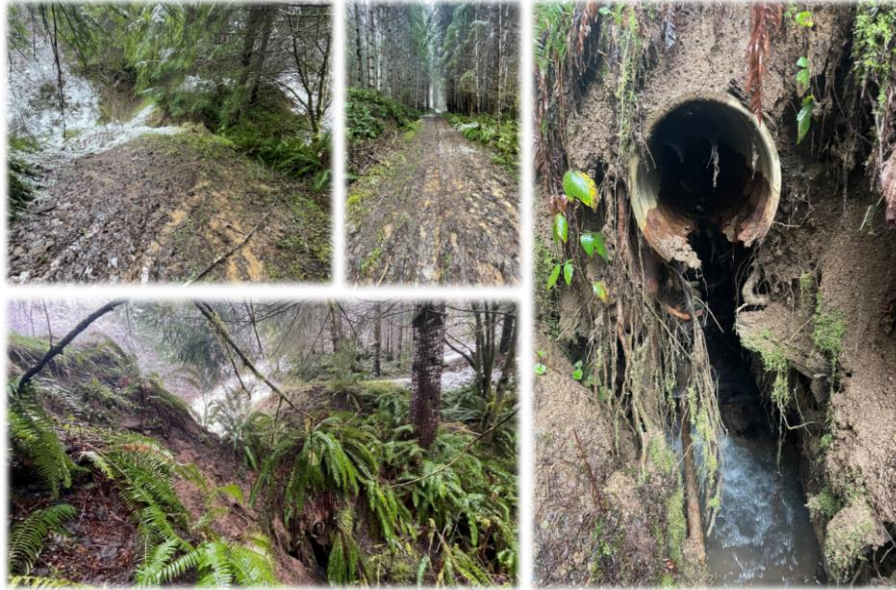
Figure 13. Photos of an abandoned road that poses a risk to waters of the state.
